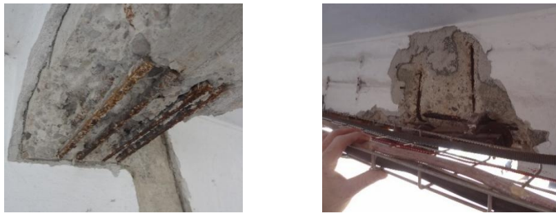
Fig. 1. Real photo of the RC beams subjected to corrosions.
